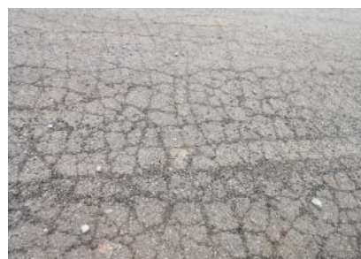
Extensive damage found along Talon Ridge Ct.
