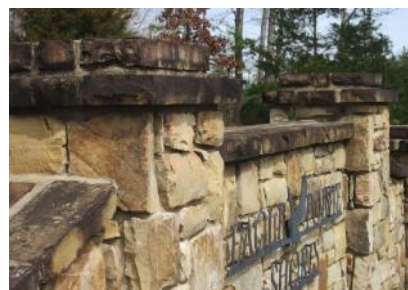
Stone will need to be cleaned.
