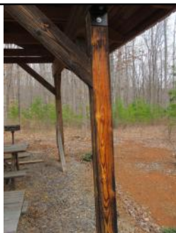
The shelters are not being maintained.
