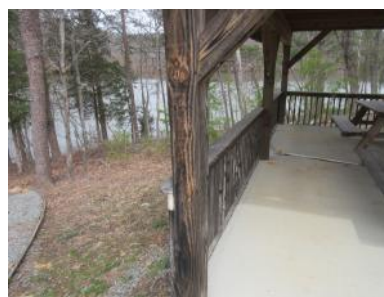
The shelters are not being maintained.
